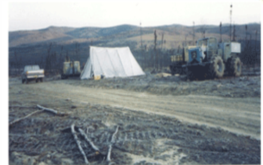
GIL EXTENSION - SUPPORT EQUIPMENT
