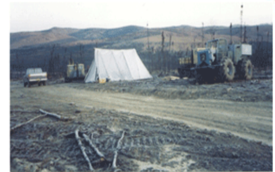
GIL EXTENSION - SUPPORT EQUIPMENT
